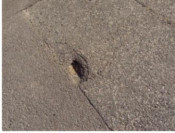
Photo 6 – uneven and broken pavement in South Road
